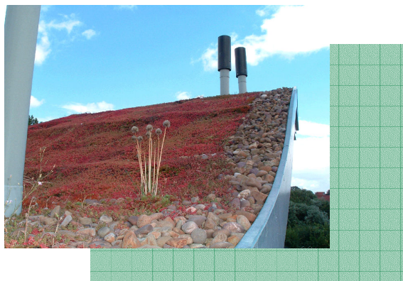
An example of a 'green roof' at the York Environmental Community Centre.
